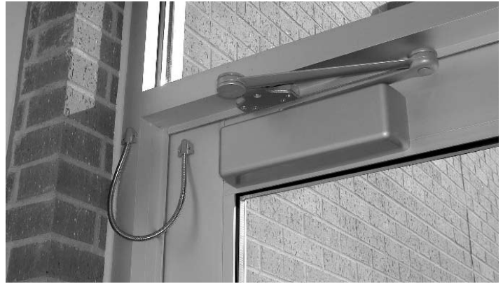
Aluminum doors and frames use loop-type power transfers, while LCN door closers ensure proper closing and latching.
