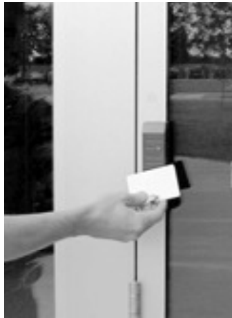
Proximity cards are used by Olathe school teachers and staff members to gain entrance to controlled doors and for after-hours access.
