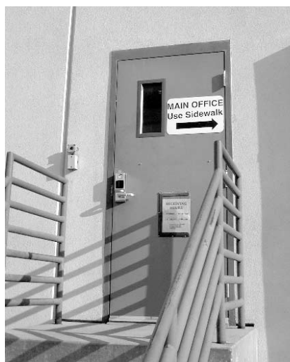
Schlage VIP open architecture integrated access control on rear entrance to the Olathe Unified School District's maintenance division combines mechanical hardware with the ability to monitor door position.
