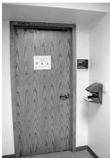
Entrance to critical areas such as this computer room at Grand Rapids Community College are protected by Schlage Recognition Systems HandKey II readers that utilize hand geometry technology to map and verify the size and shape of a person's hand in less than one second.
