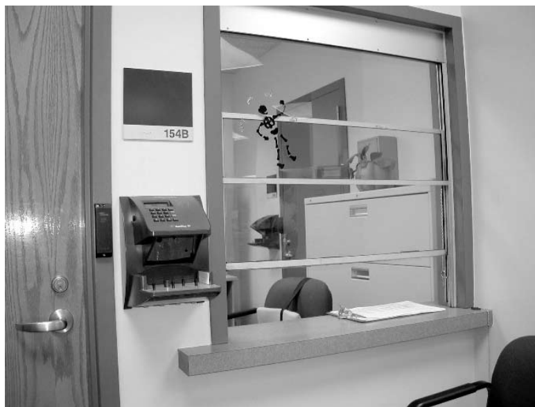
Two HandKey readers protect the college's records and financial assets. One controls entrance to the Cashier's office, while a second, visible next to the door inside, protects the vault.
